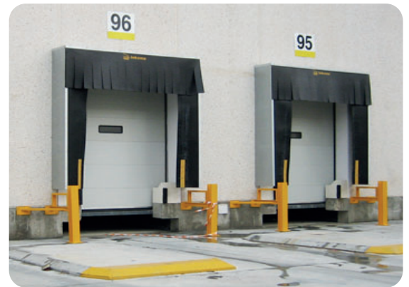
Fixed Dock Shelters installed directly at the facility.
