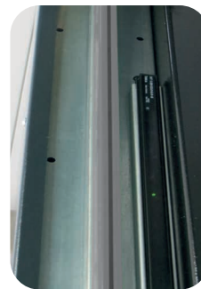
Photocell Curtain and Guide Rail.
