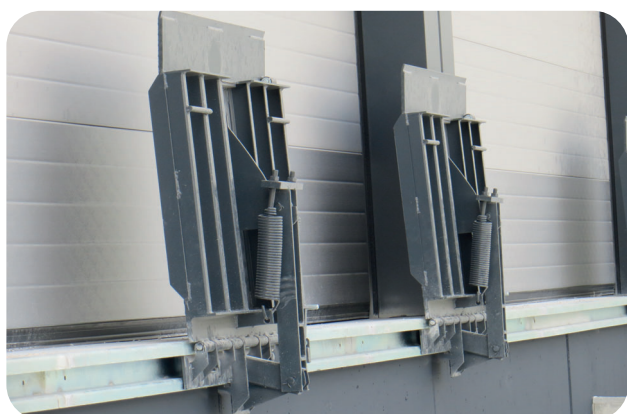
A1 installed on loading dock.
